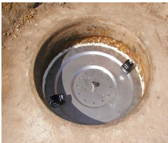
3) WHEN WORK IS COMPLETE, ALIGN EYE BOLTS WITH THE SLOTS IN THE INNER COVER, REPLACE THE INNER COVER, AND SECURE THE PADLOCKS.
