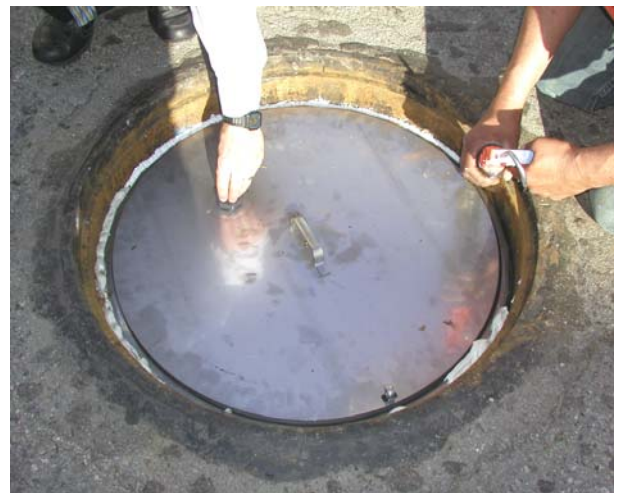
FOR MANHOLES WITH OPTIONAL ODOR CONTROL RING WITH PRESSURE SEAL, BEFORE REMOVING THE INNER COVER, AIR TEST FIRST USING THE BULKHEAD.
